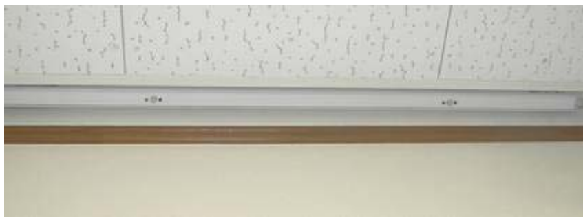
Infra-red sensors at each room entrance, which detect in and out of people.
